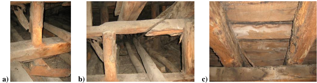
Figure 2.2a,b,c. Massive timber roof elements with different stages of wood destruction
