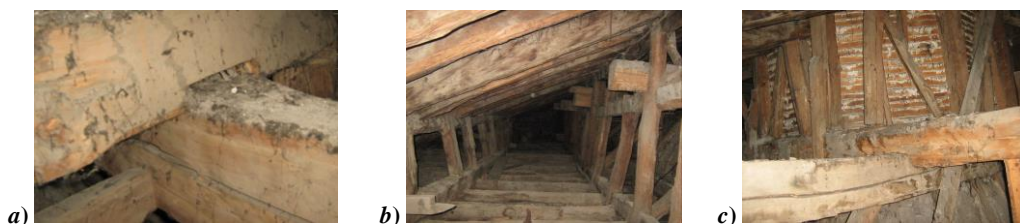
Figure 3.3a,b,c. Torsion of beam, horizontal displacement in the top of columns: a), vertical displacement of beam – caused the creep: b), and cracks in the beam: c)
