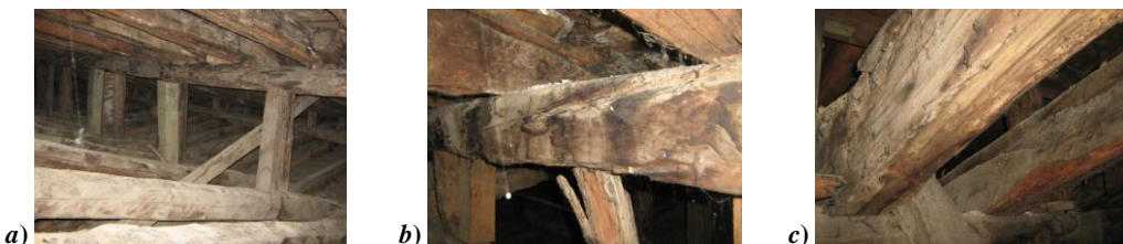
Figure 2.1a,b,c. Moisture in purlins in axis B and D
